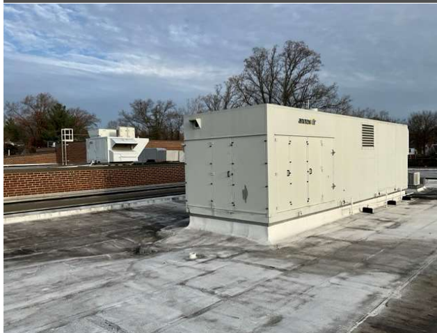
25 - ROOFTOP MECHANICAL EQUIPMENT
