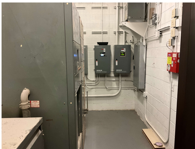
27 - MAIN ELECTRICAL ROOM
