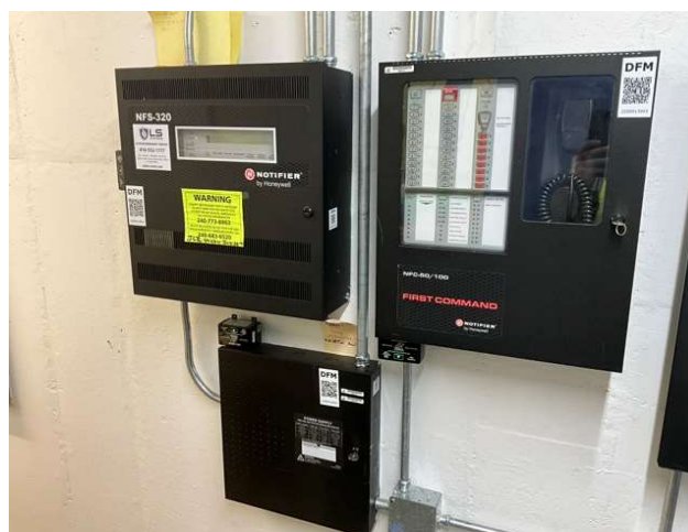
30 - FIRE ALARM PANEL
