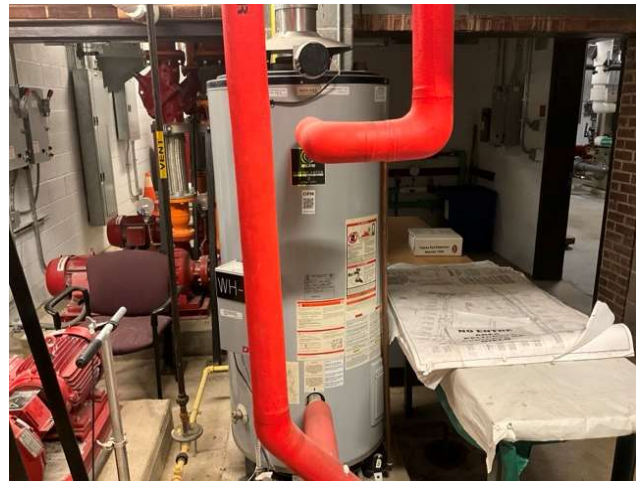
22 - DOMESTIC HOT WATER SUPPLY
