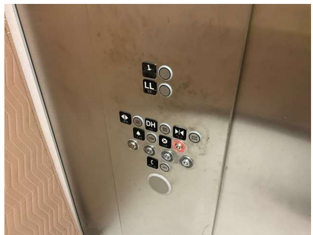
18 - ELEVATOR CAB PANEL
