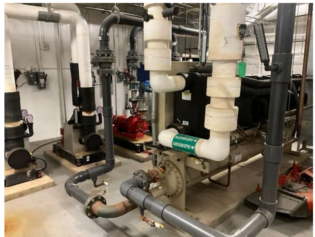
24 - MAIN MECHANICAL ROOM
