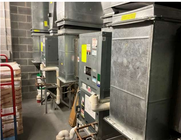
23 – WATER SOURCE HEAT PUMPS
